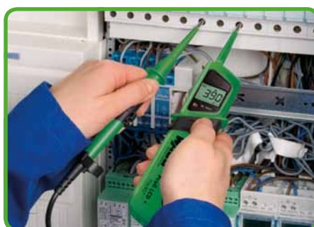
Voltage testing in switchgear cabinet.
