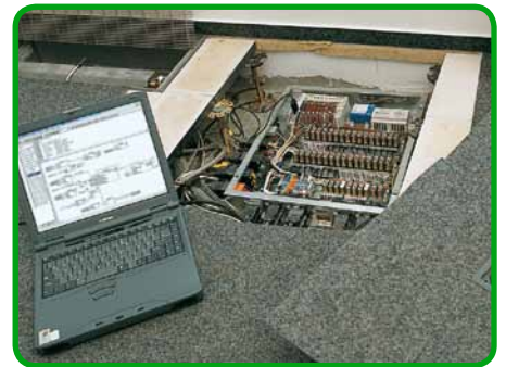
Under-floor distribution boxes
