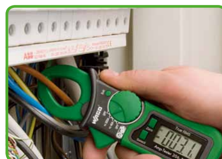
Current measurement in switchgear cabinet.
