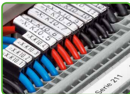
Conductor marking using marking sleeves.
