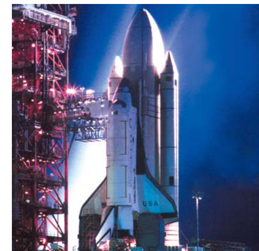
RAB explosionproof fixtures light the Space Shuttle launch tower at the Kennedy Space Center.
