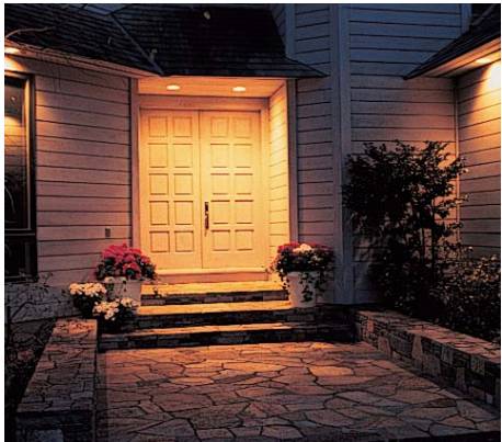
Smart Box controls 500 watts of front door lighting. (Hint: Look on the wall to the left of the door.)
